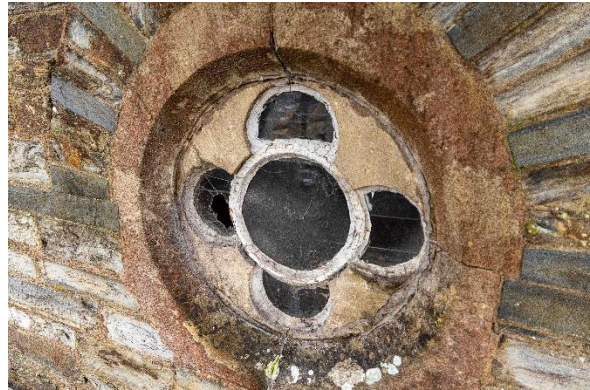
19 Feb 26 – the starting point – broken glass.
