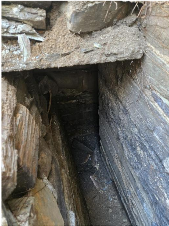
5 May 26 – 5-foot deep culvert discovered.
