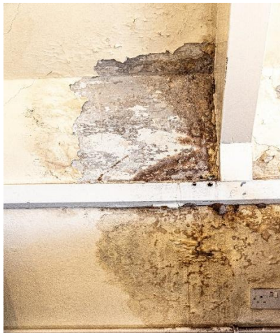
Damp and fungi in the upper room
