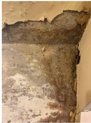
Damp outside the upper room
