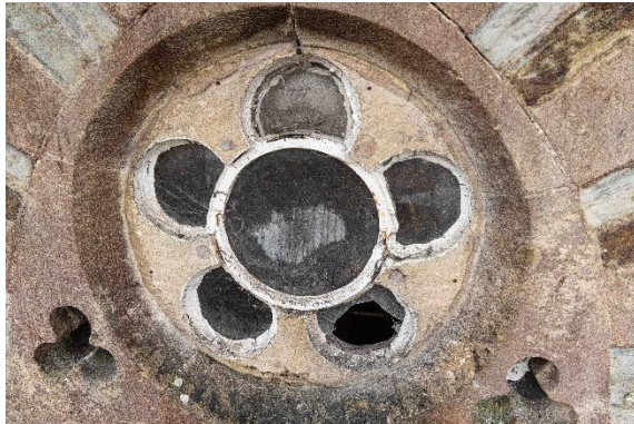
19 Feb 26 – the starting point – broken glass.
