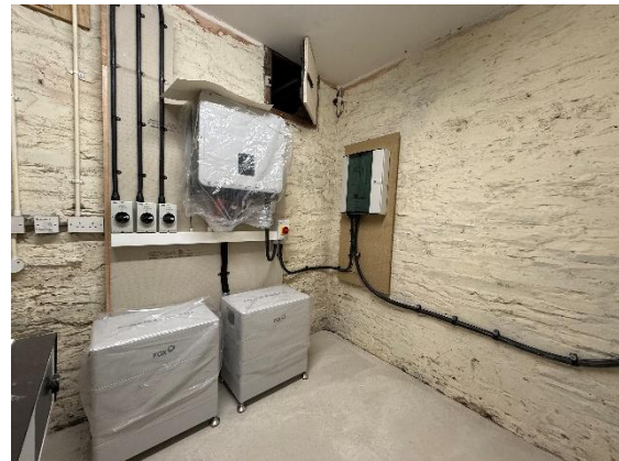
The finished system – 40 kWh batteries resting on new concrete base in the plant room.
